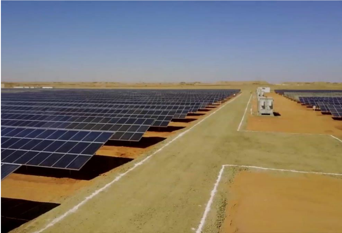
PV Solar in Egypt
