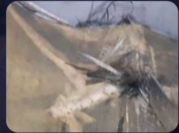
FLASH OVER DAMAGE
