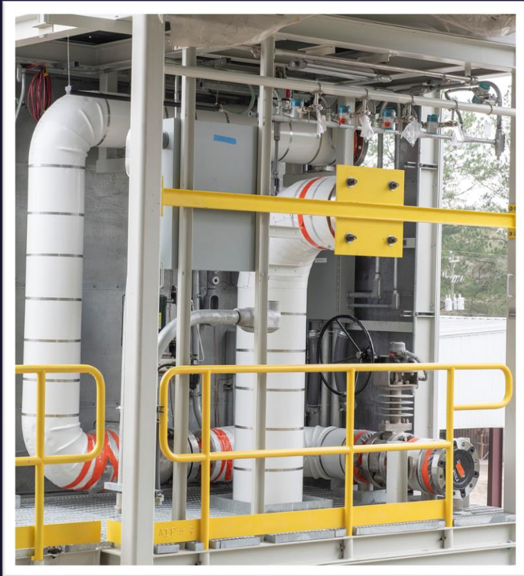
Open Bays for GT Access
