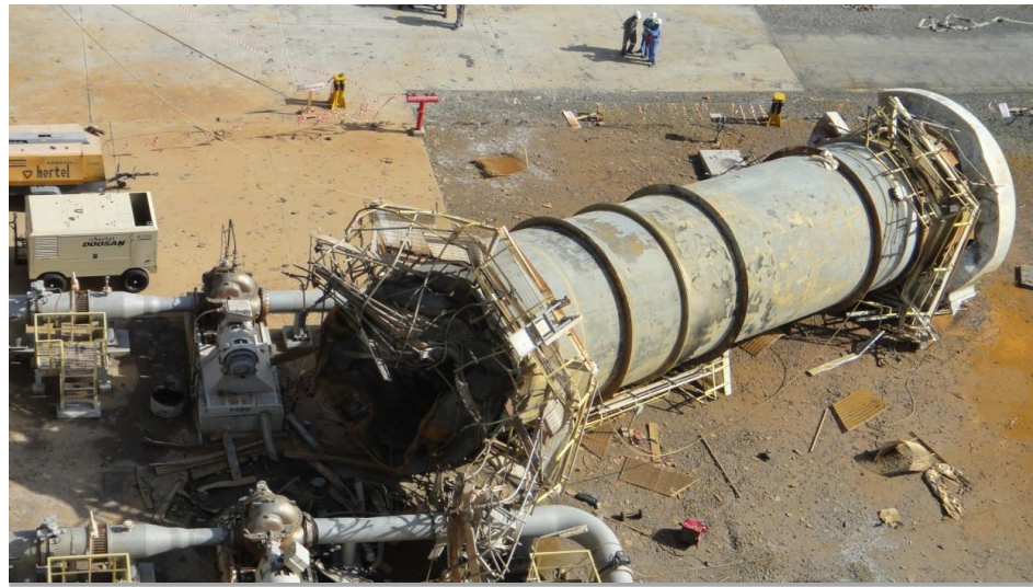
Fire in a wet gas scrubber absorber unit
