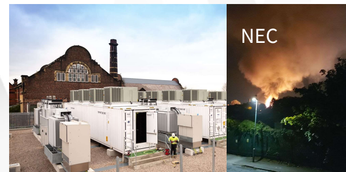
Carnegie Rd Battery Fire
